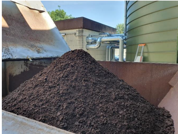
Figure 5: photograph of dewatered excess sludge for use as biogas plant feedstock
